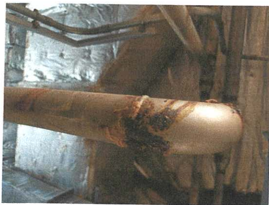
The elbow corrosion
