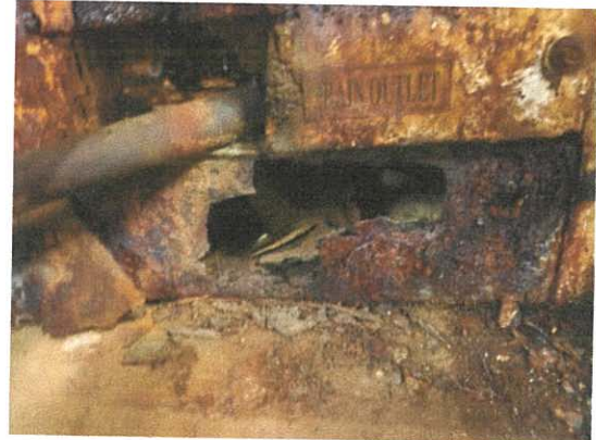
The corroded structure
