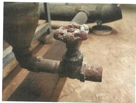
The valve condition
