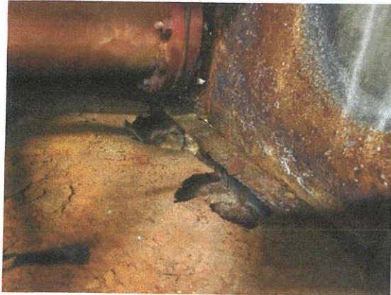
The corroded structure
