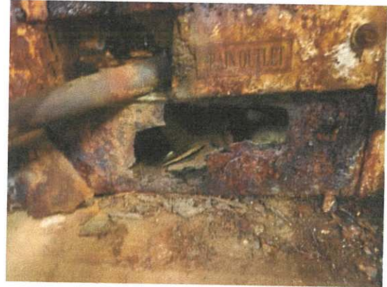
The corroded structure
