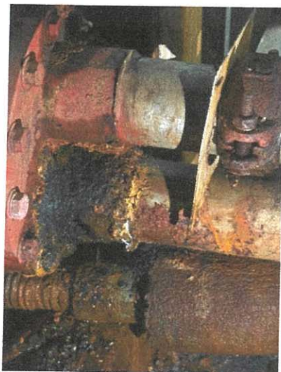
The pipe damage
