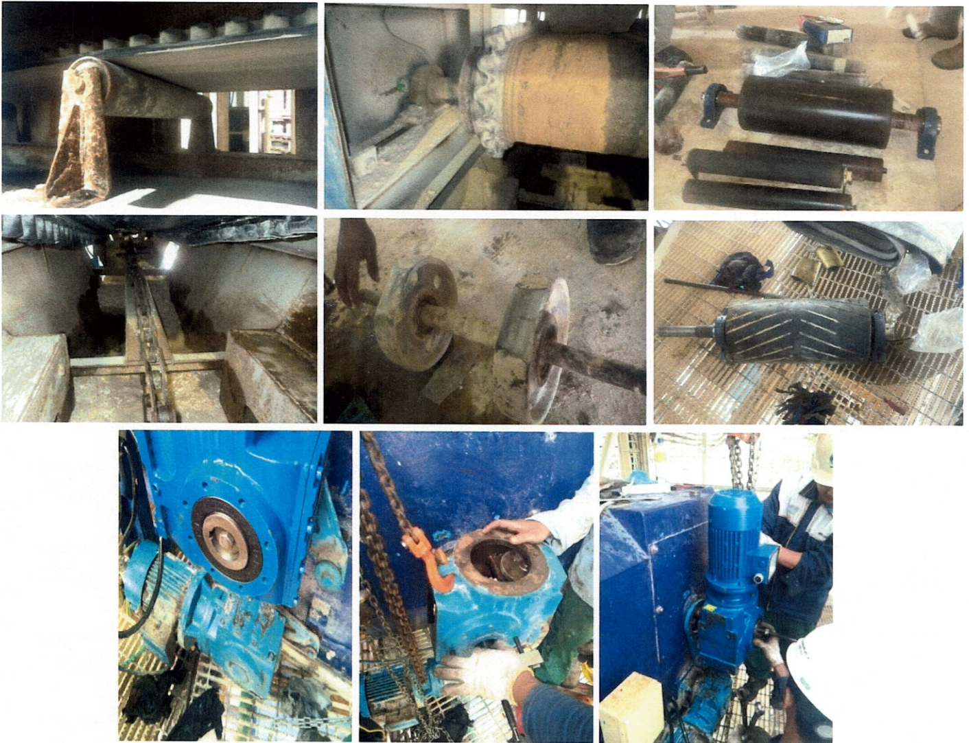
Limestone weight feeder A&B maintenance
