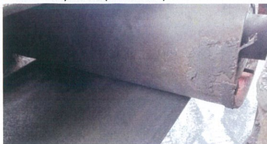
Boom Conveyor SR A (Area Bucket)
