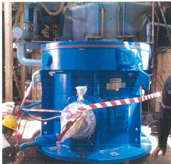
Coal Pulverizer Reduction Gear VRP-125
