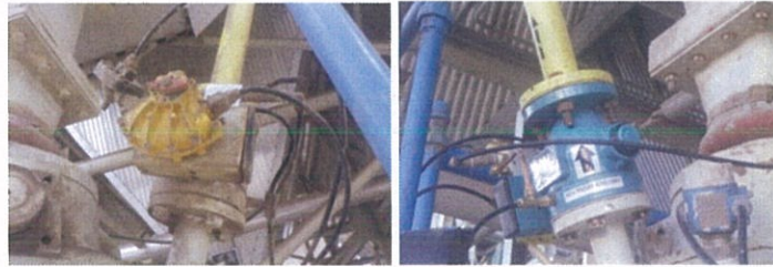
DN50 Dome Assembly: 1. ESP Field 1&2 vent valve
