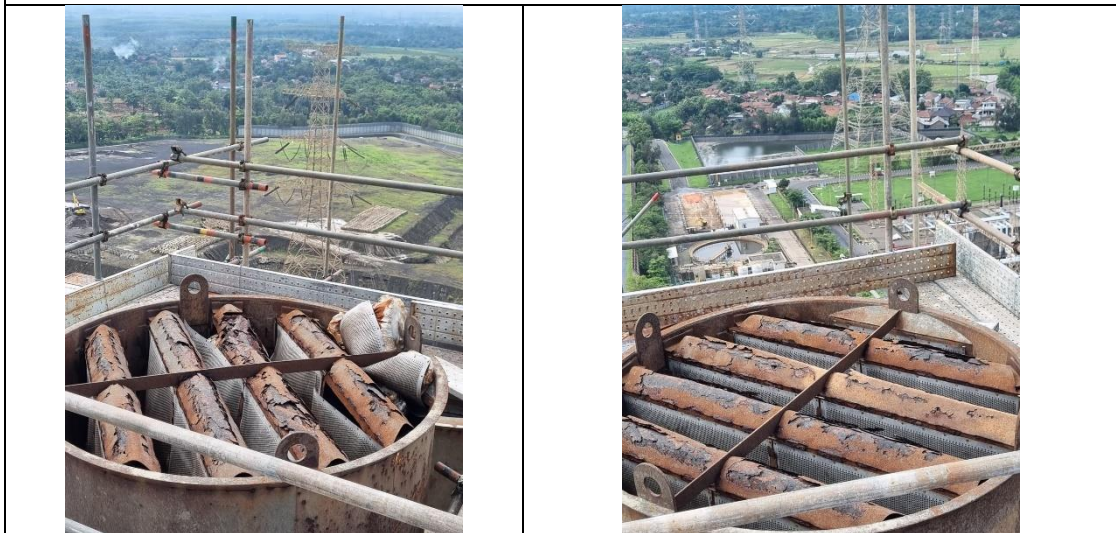
Reheater Inlet Safety Valve Silencer A and B
