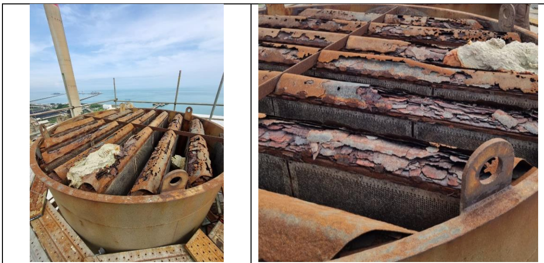
Superheater Outlet Safety Valve Silencer A
