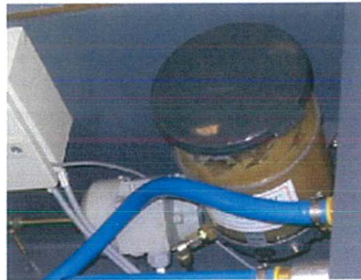
Filter element & oil indicator
